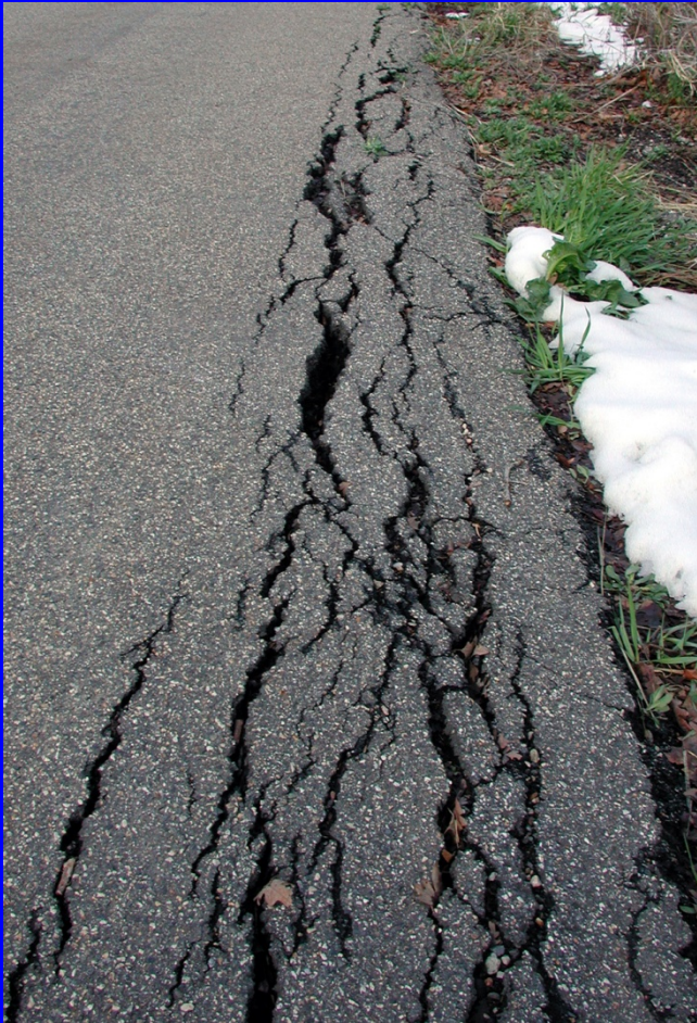
Extension fractures at the edge of a paved road. Pavement is saturated with fractures and additional strain will be accommodated by the coalescence of existing fractures.
