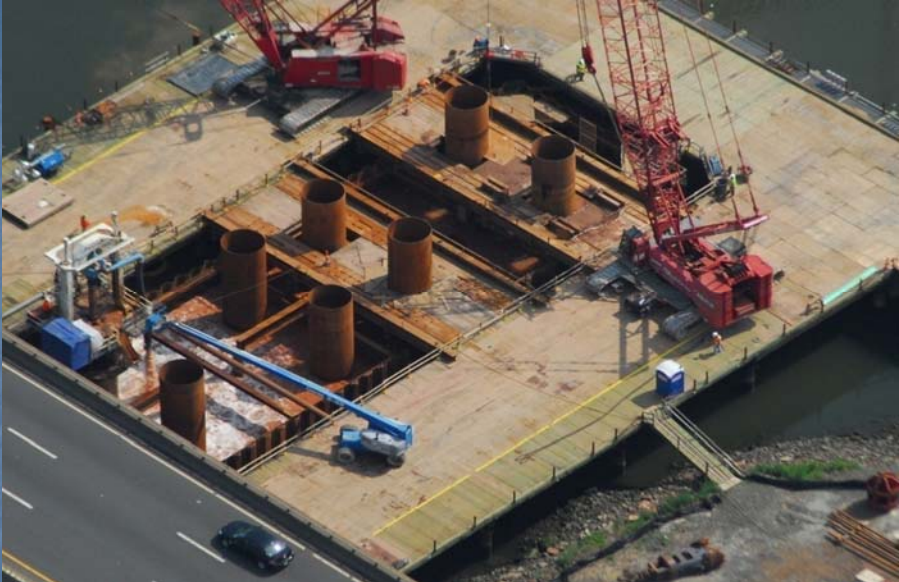
RCD drawing water from river and expelling drill cuttings into marine enclosure
