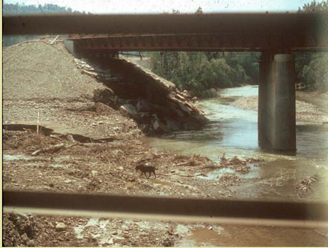
Bridge Abutment Scour
