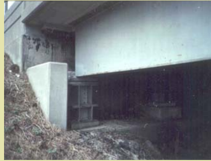
Bridge Abutment on Piles - 30 inches of Settlement over 10 years
