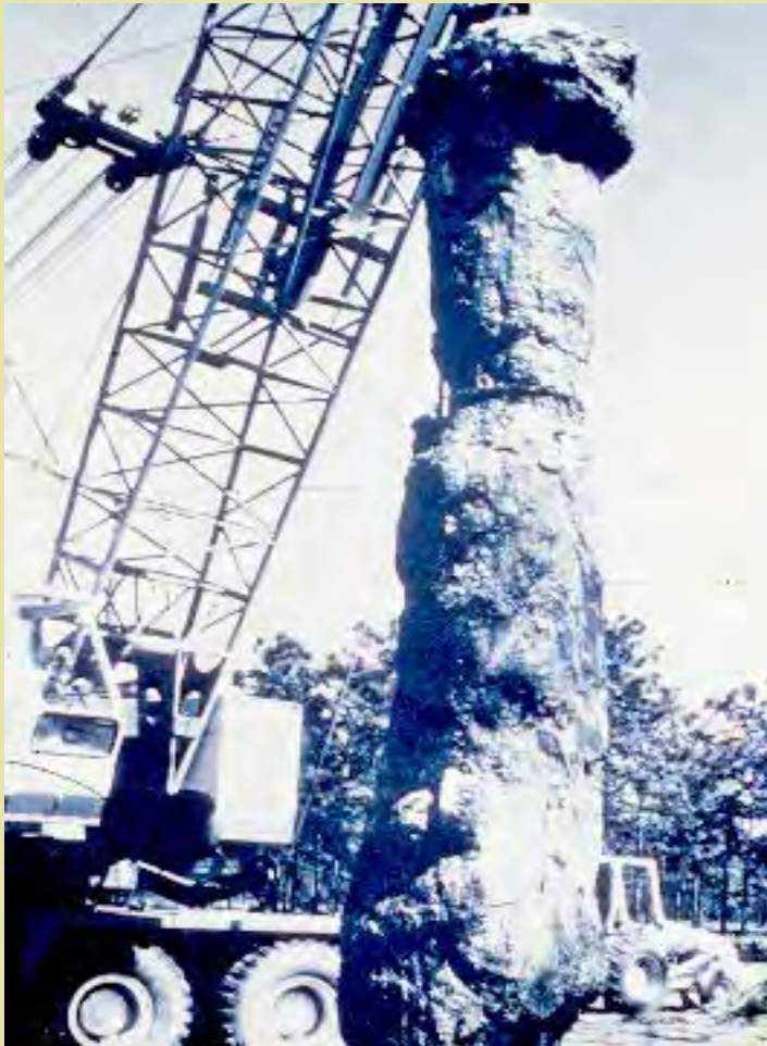
Poor Slurry Job
