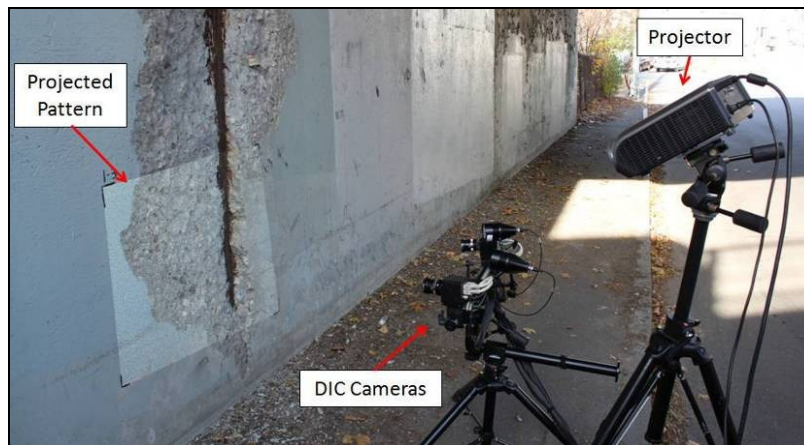
Figure 3.2 Experimental setup for projected pattern measurement to quantify spalling on a bridge in Lowell, MA
