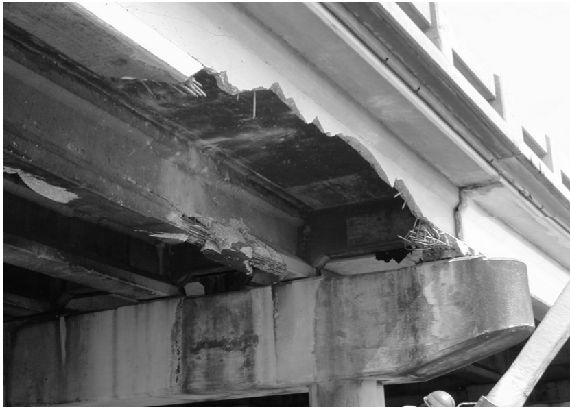
Structurally deficient bridge
