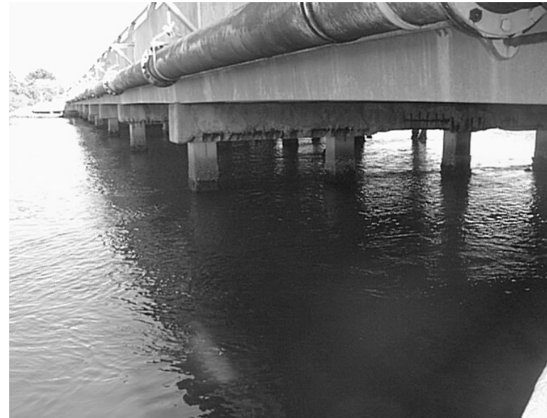
Functionally obsolete bridge
