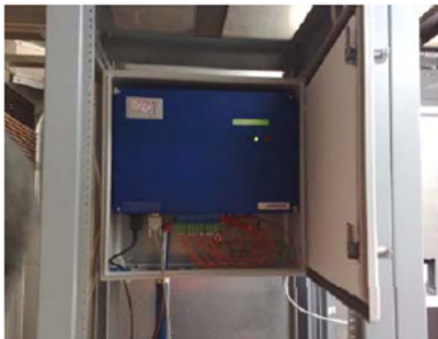
(e) SOFO Fiber Optic Sensor Datalogger
