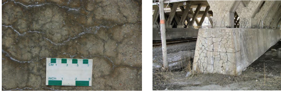
(a) Exudation of ASR gels from cracks (b) Severe cracking of bridge column
